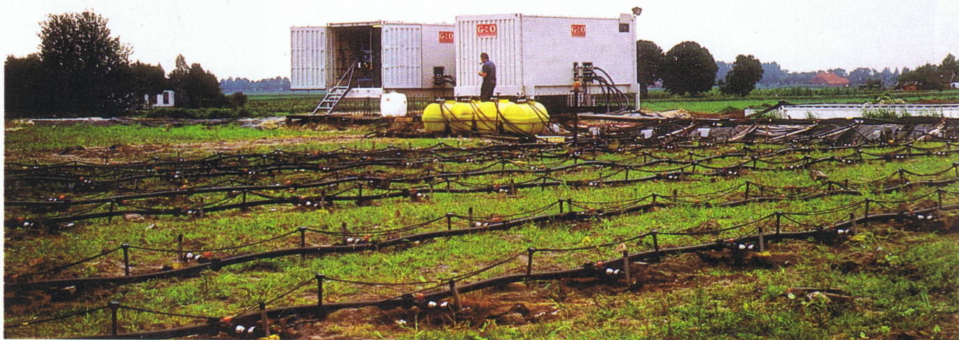
Electro-Reclamation in practice — Anode-series with circulation system and electricity supply. Cathodes are installed horizontally in between anode rows. In the background are containers for conditioning and treatment of electrode-solutions.
